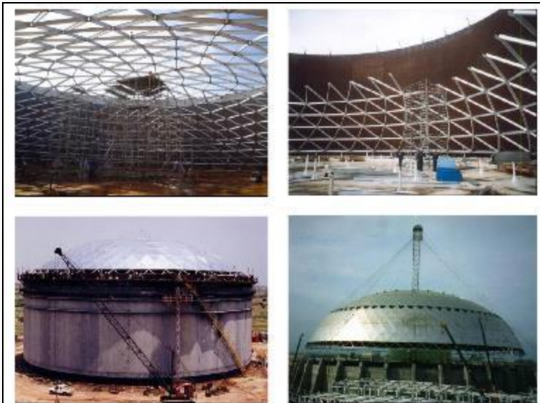
Figure 2.2.1 - Geodesic domes can be built on the ground and lifted into place or built directly on the existing floating roof tank and winched into place. A variety of methods are available for erection, including "jack stand" erection (top), "grip hoist assembly (bottom left) and "lower assembly (bottom right).
